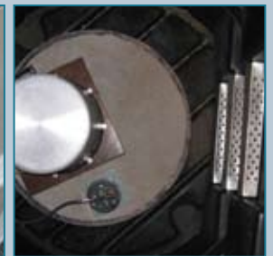
MANHOLES FOR INSTRUMENTATION
